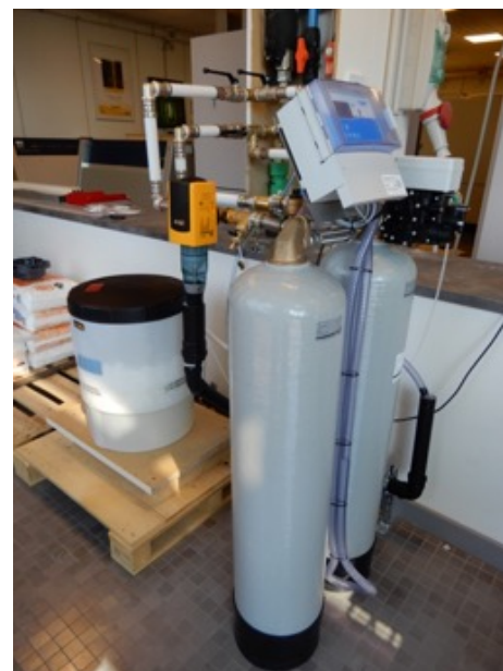
Picture 1. Softening plant
